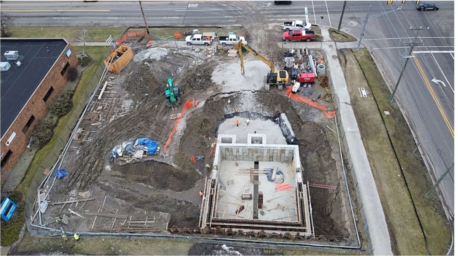
Figure 14 – Macomb Township Bio-Filter Media Chamber
