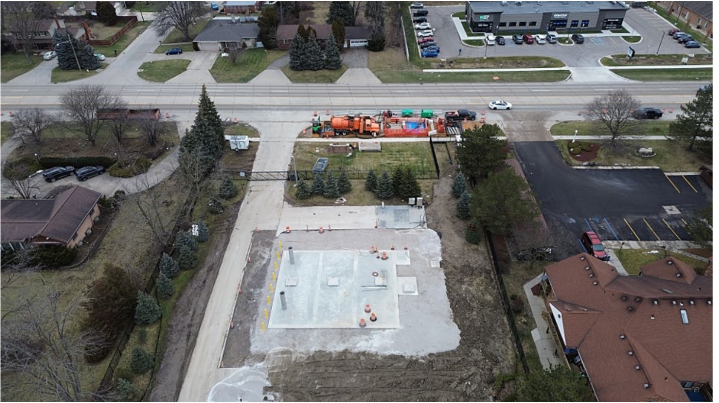
Figure 12 – Fraser Bio-Filter Access
