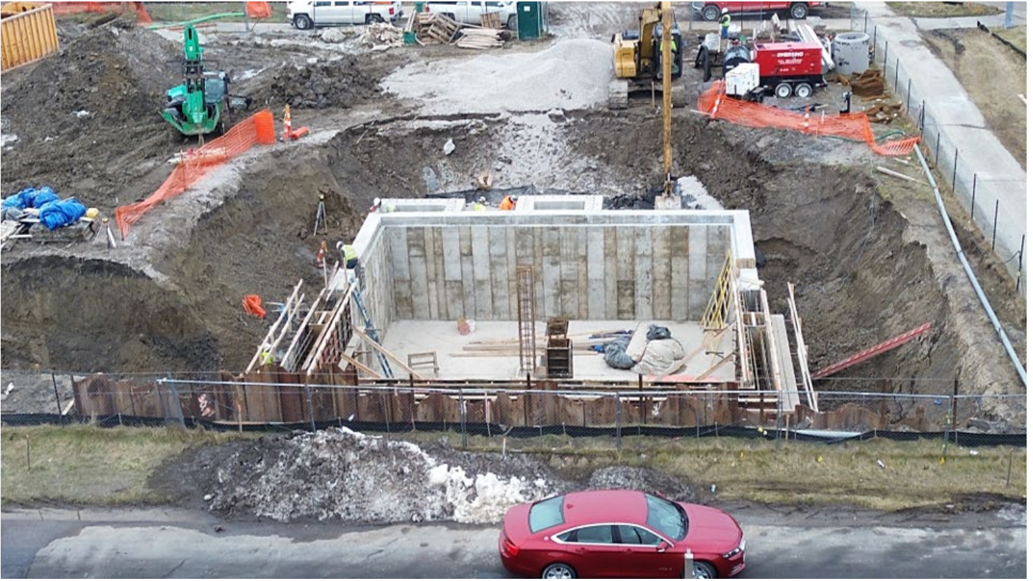
Figure 13 – Macomb Township Bio-Filter Media Chamber
