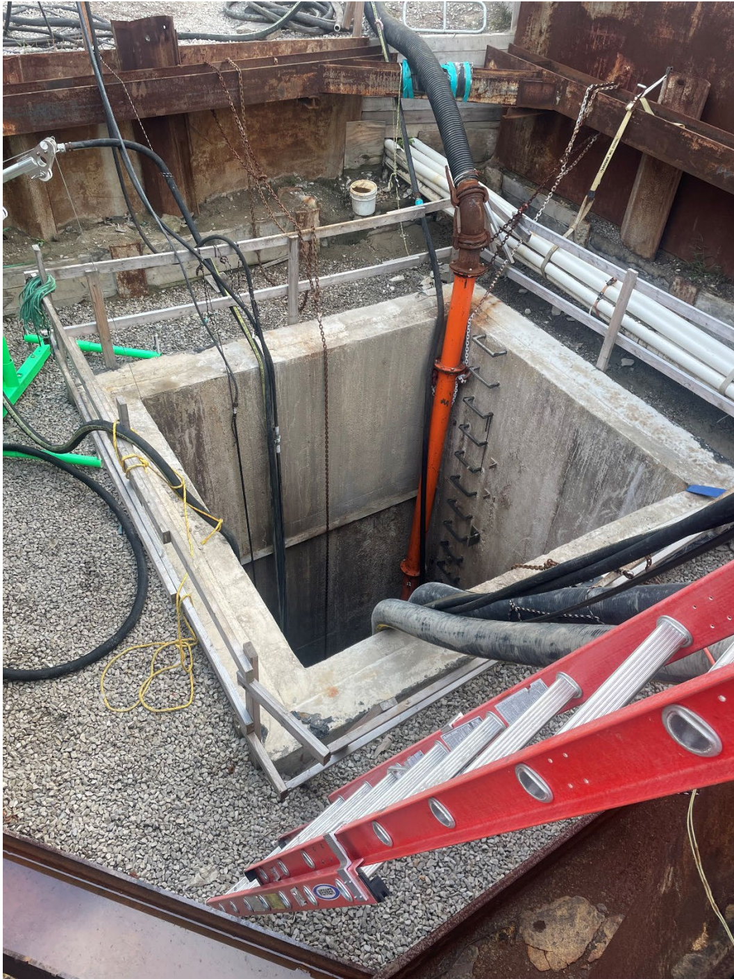
Figure 10 – RAI Curve Cleaning Setup at CS-2
