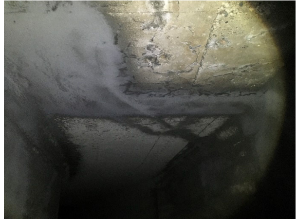
Figure 4 – 9MD ceiling damage – after patch
