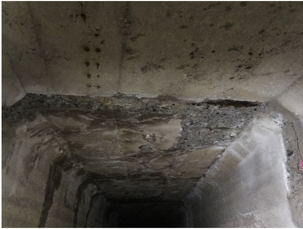
Figure 3 – 9MD ceiling damage – after demo, before patch
