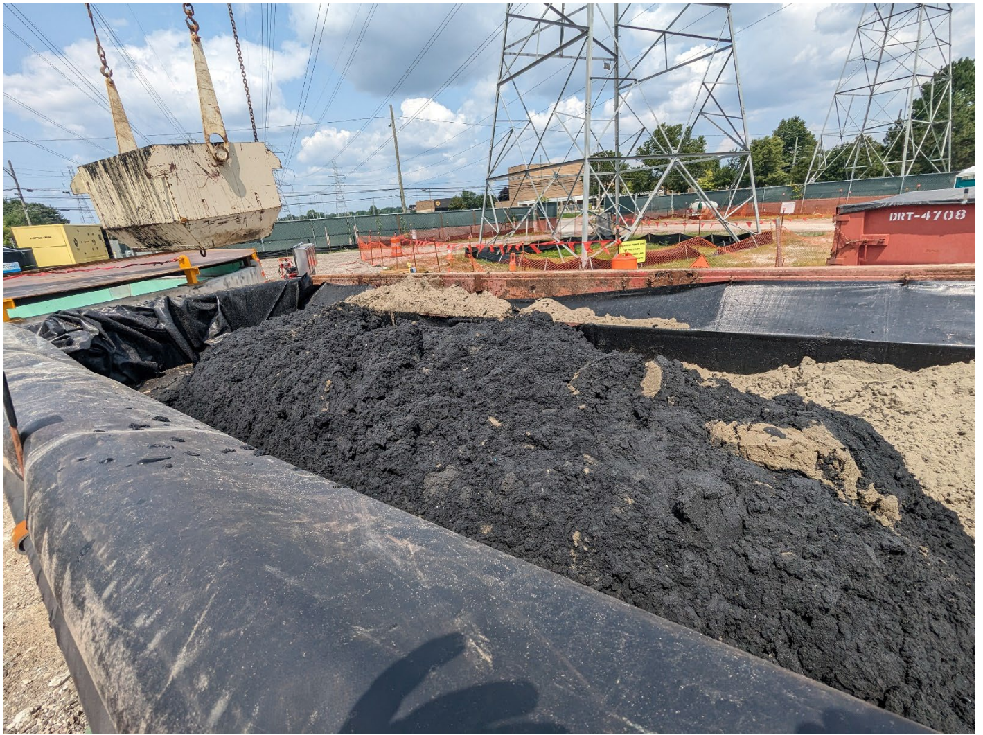
Figure 4 – Debris Coloration Immediately after removal from Interceptor
