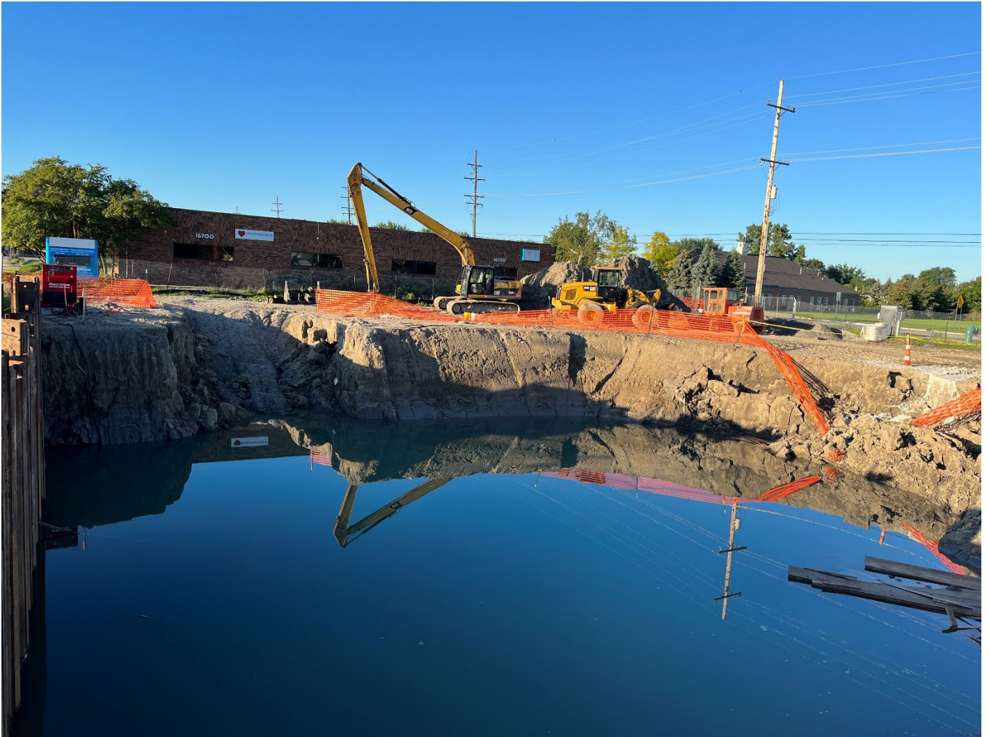
Figure 15 – 21 Mile & Garfield – Groundwater Infiltration
