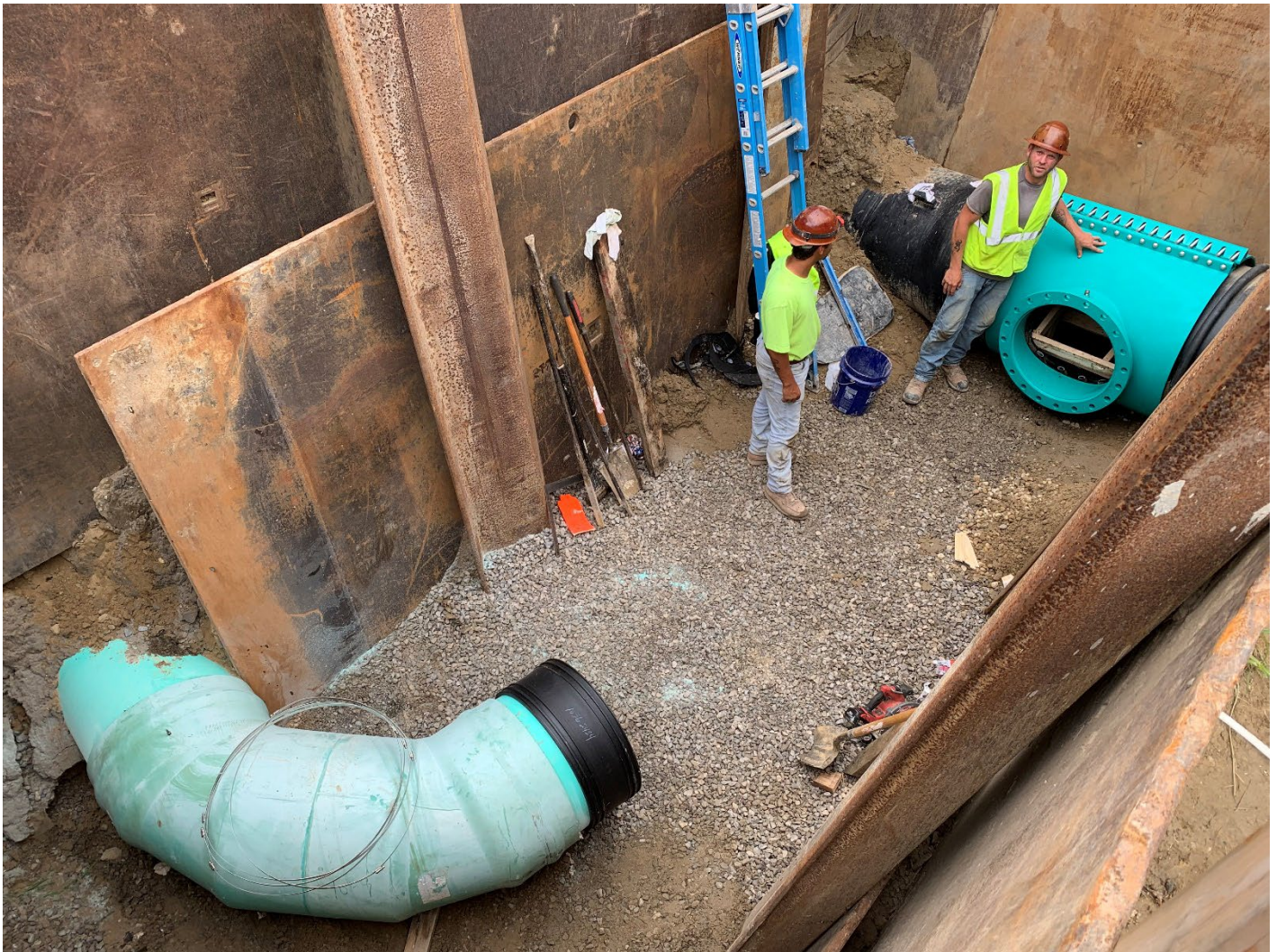
Figure 6 – FAD Connection at existing Bio-Filter line
