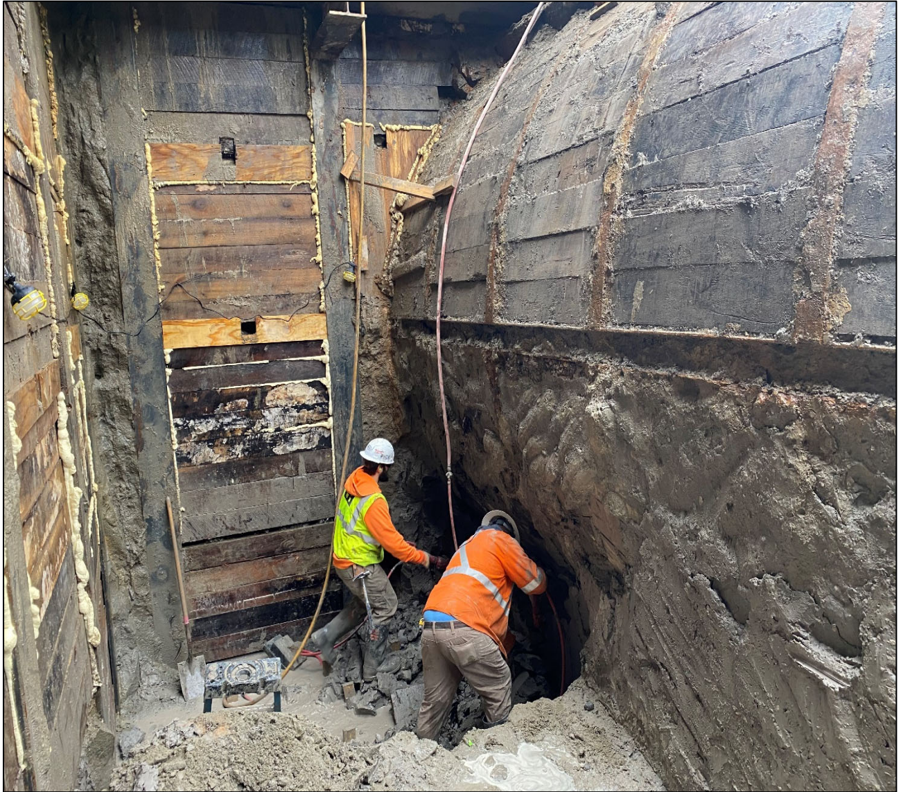
Figure 4 – Undermining South Side Tunnel at West Wall
