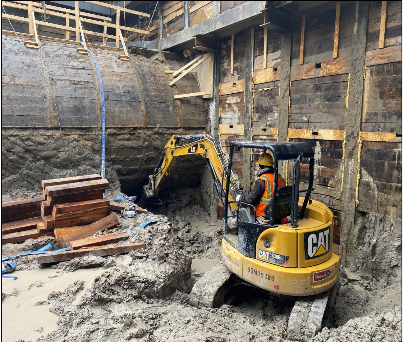
Figure 3 – Undermining North Side Tunnel at West Wall
