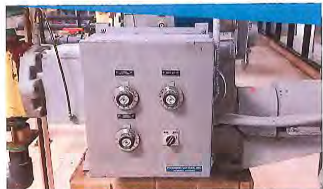
The chemical feed pumps at both Chapaton and Martin Basins require upgrading because replacement parts are no longer available from suppliers.
