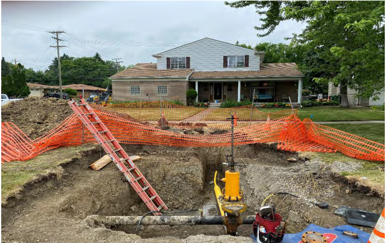
Figure 3 – Natural Gas Bypass at Beaconsfield and Oak
