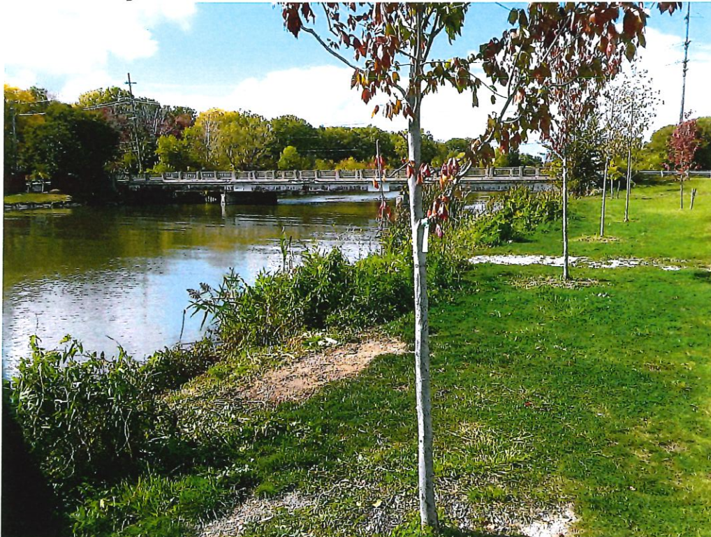
Photo 10: Area of plantings/ shore stabilization. Erosion control fabric and soil appear to have been placed over riprap.
