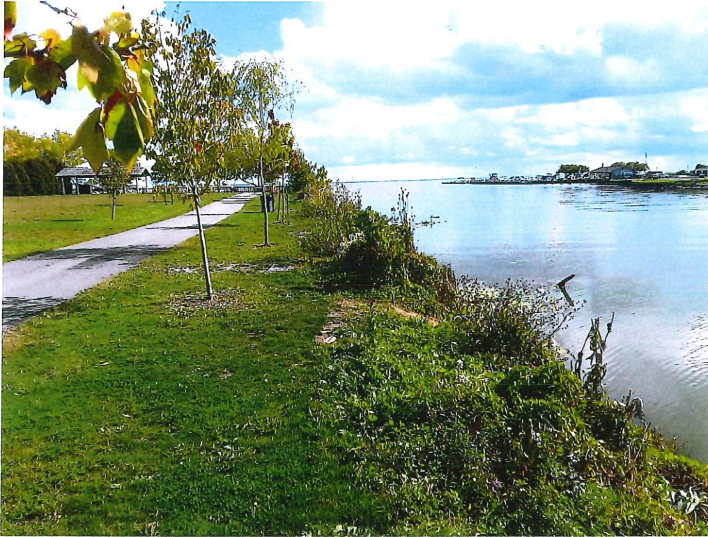
Photo 7: Left bank of channel near Lake St. Clair. Area of erosion. Bank restoration recently completed, but sinkholes and bare areas of soil noted.
