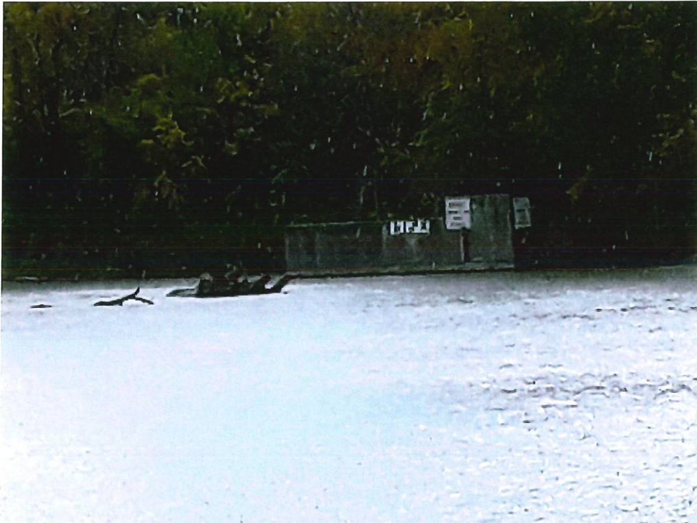
Photo 3: Left (north) abutment wall of weir. County periodically removes woody debris from the weir.
