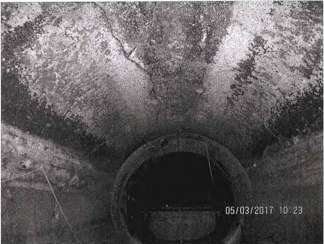
11 foot dia. interceptor crown fractures looking downstream toward the manhole at station 85+95
