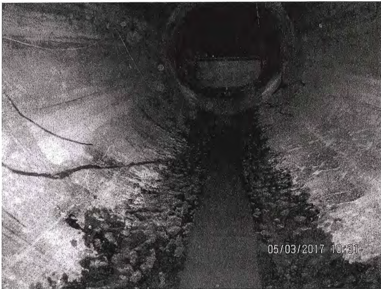
11 foot dia. interceptor invert fractures looking downstream toward the manhole at station 85+95
