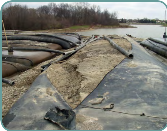
Too much sediment split this filter bag. Bags should not be filled more than 1/2 full of sediment.
