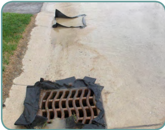
The inlet at the top of the picture is protected with a traditional geotextile fabric. The inlet at the bottom is protected with an inlet filter bag.
