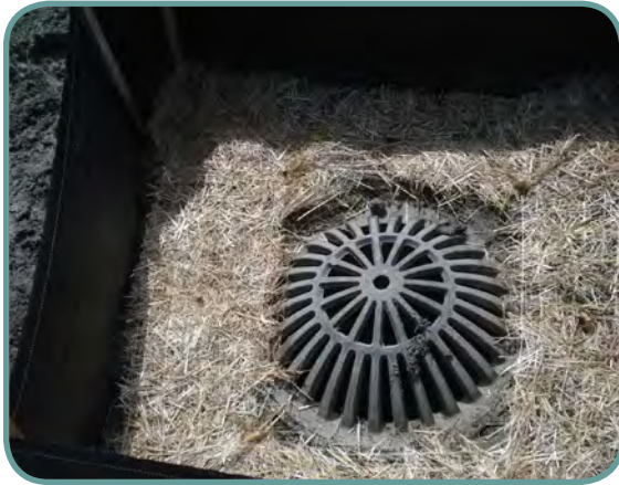
Good application of silt fence to protect an area inlet. Use wire fence backing to reinforce frame, or diagonal bracing across top of stakes. Make sure the fence is trenched in to prevent bypasses or undercutting.
