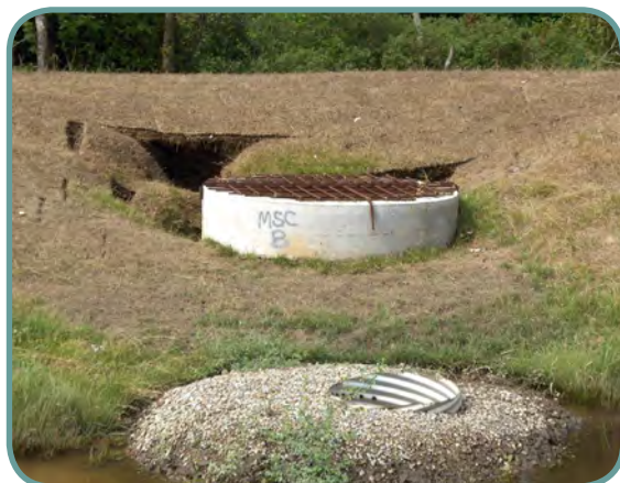
Insufficient soil compaction led to a slope failure on the bank of the detention basin. The CMP outlet structure (pictured in the foreground) is missing a bar grate cover.
