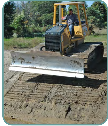
The photo shows a good example of surface roughening. The dozer is tracking up and down the slope creating grooves in the soil perpendicular to the direction of flow down the slope.
