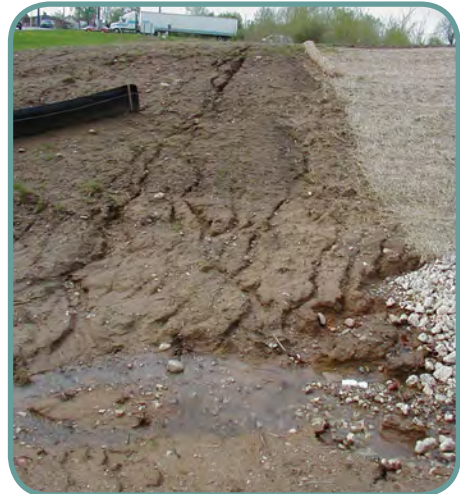
The slope on the right is protected with properly installed mulch blanket. The slope shown on the left is unprotected. Rills and gullies have formed on the slope. The silt fence is not placed parallel to the contour or the slope.
