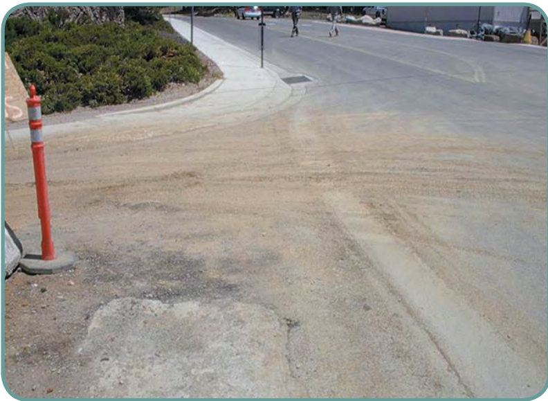
Construction access drives are required before clearing and grading work begins. Access drives must be maintained until the site is stabilized. Inspections should note whether mud is being tracked onto paved roads. This photo shows an example of a construction access drive that is not properly stabilized.
