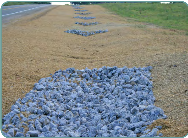
Wide and relatively flat ditches can be protected with seed and mulch. Steeper ditches (e.g., slopes of up to 10% and more in some cases) can also be seeded if turf reinforcement mats are used. Check dams can help to control downcutting in drainage ditches before grass is well established.
