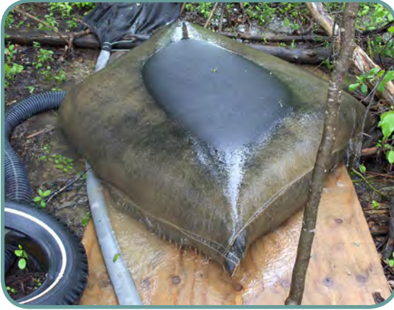
This is an example of a filter bag in service. A stable and level bed of gravel should be used instead of a plywood base.
