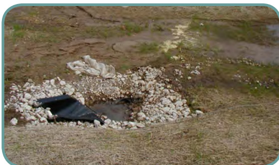
This photo shows an improperly sized and constructed energy dissipater.
