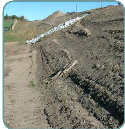
This photo illustrates improper surface roughening. The grooves are parallel to the direction of flow. Notice the sediment fines being deposited at the base of the slope due to erosion.
