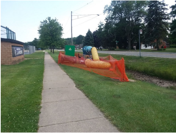
Figure 5 – Ventilation Equipment Set-up
