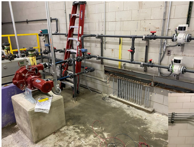
Figure 2 – New hose pumps, plumbing, valves and flow meters
