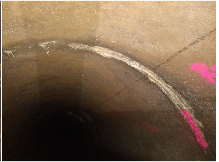
Figure 11 - Infiltration at Construction Joint
