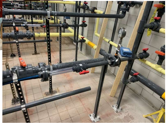
Figure 5 – New disinfection feed piping and supports (adj. to existing)
