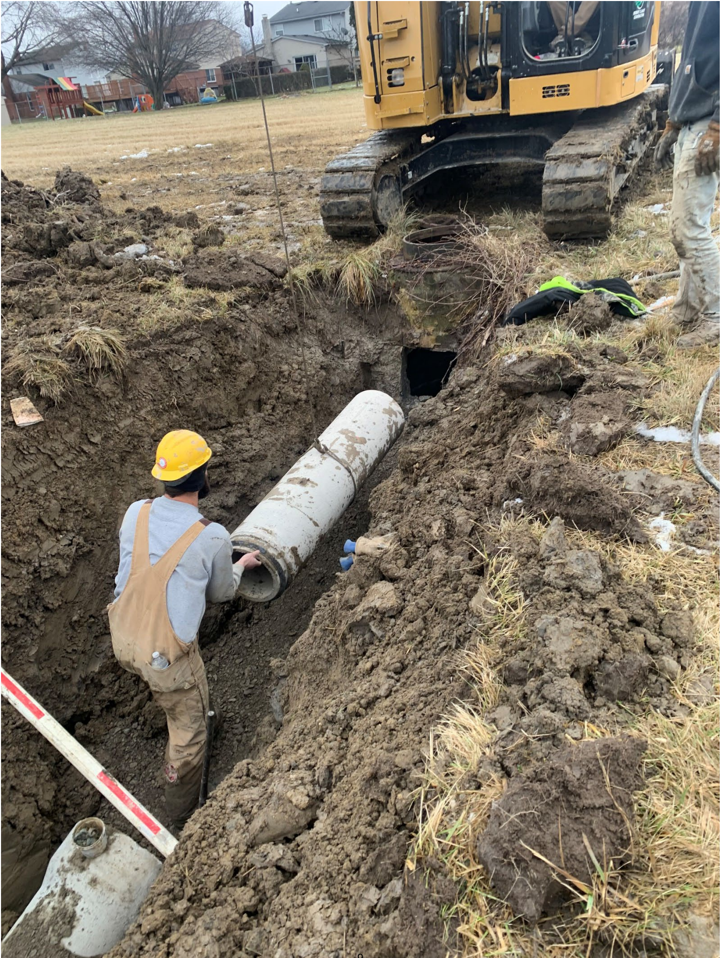
Sinkhole #2 300ft. West of Sinkhole #1 on West Side of Ivy Street
